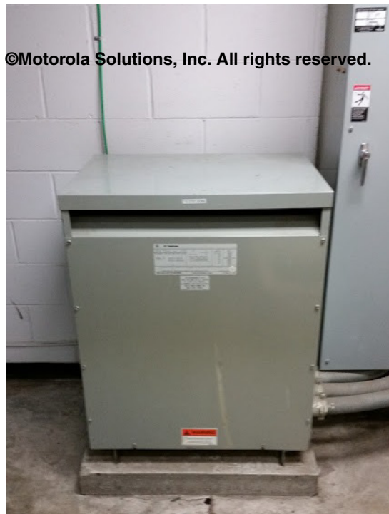
Figure 5-79 Example of Transformer
