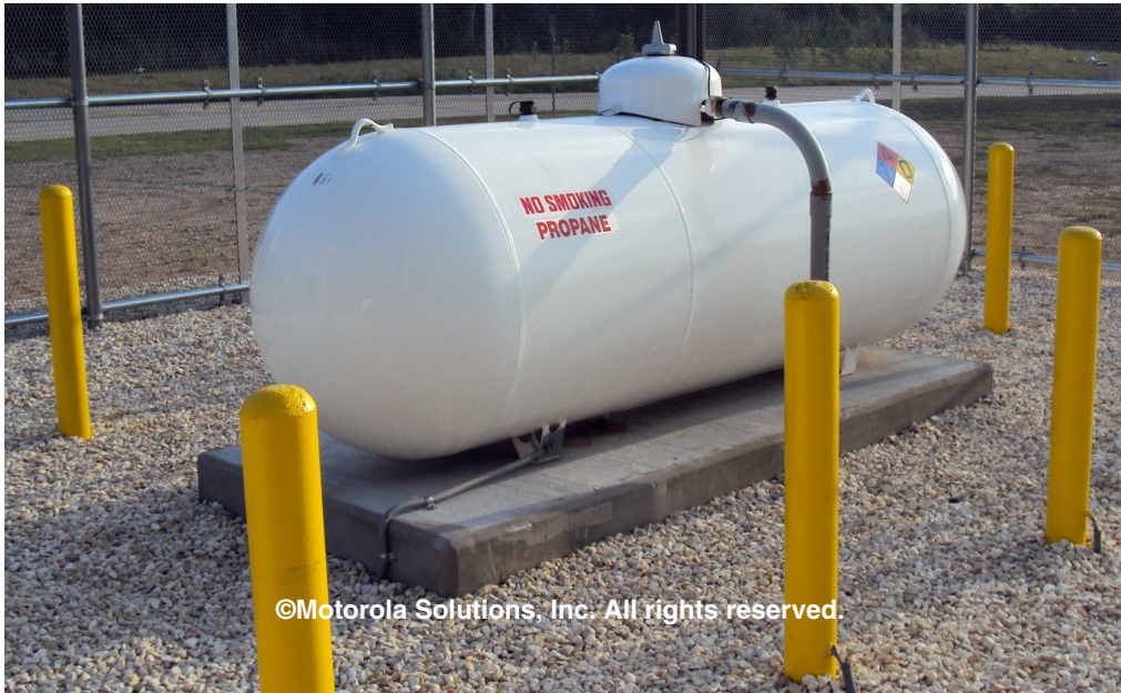
Figure 4-92 Example of Above-Ground Propane Tank Grounding
