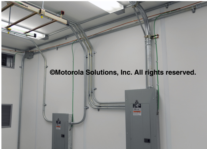
Figure 5-103 Example of Bonding Electrical Panelboard to Internal Perimeter Bonding Bus
