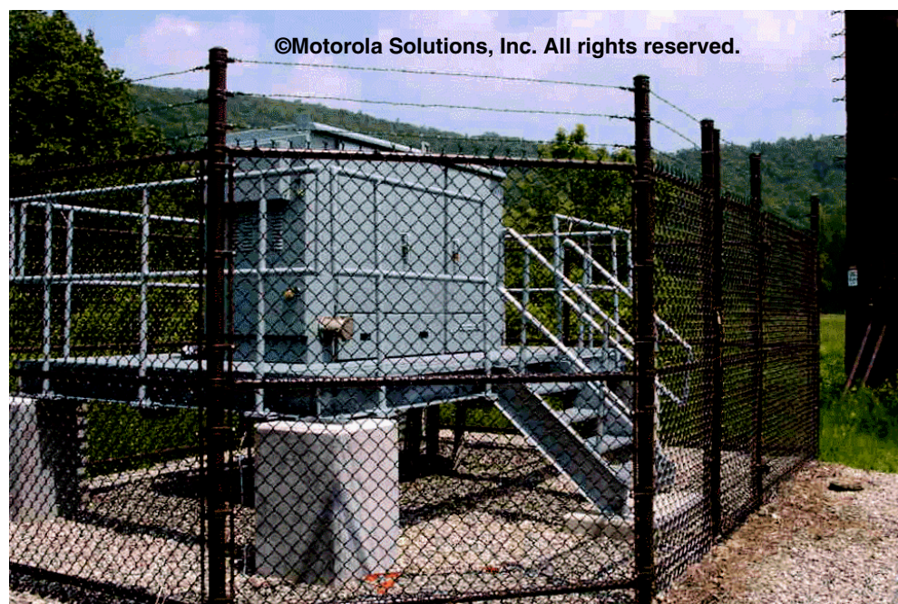
Figure 3-3 Typical Outdoor Enclosure Cabinet on Raised Platform
