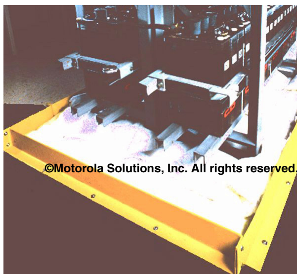
Figure 6-18 Example of Battery Spill Containment System
