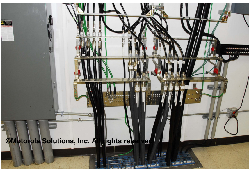
Figure 5-23 Wall Supported Secondary Bonding Bar at a Floor Level Communications Cable Entry Port
