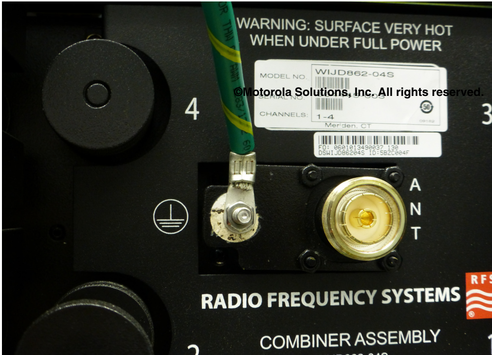
Figure 5-87 Example of Equipment Bonding - Antenna Combiner
