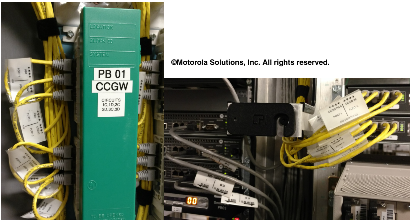
Figure 9-51 Examples of Cable Labeling
