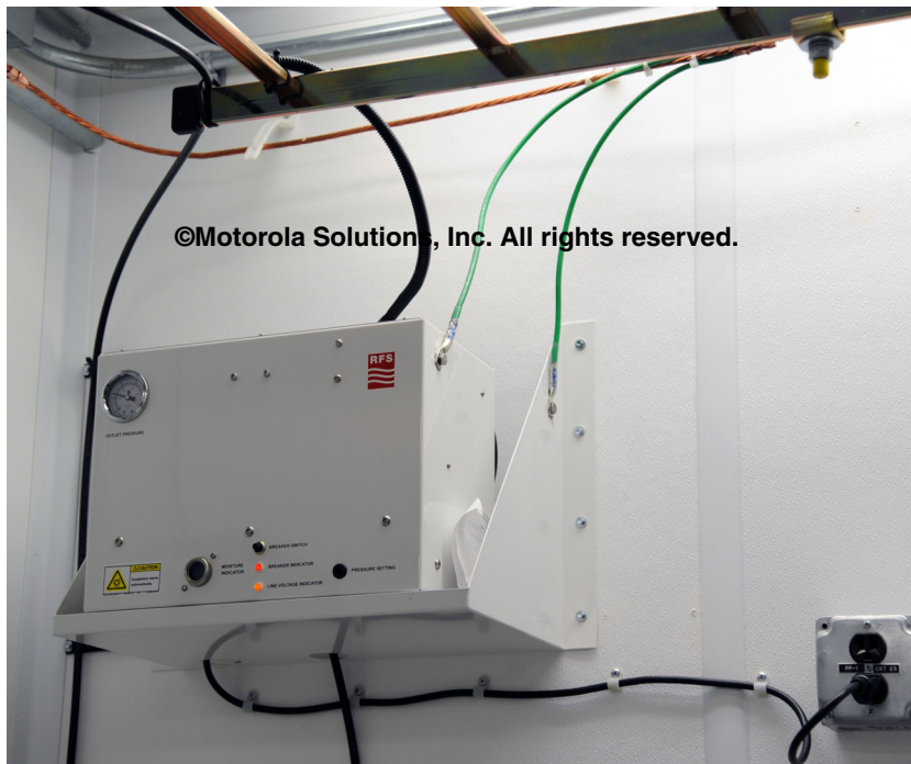
Figure 5-107 Example of Bonding Dehydrator and Shelf to Internal Perimeter Bonding Bus
