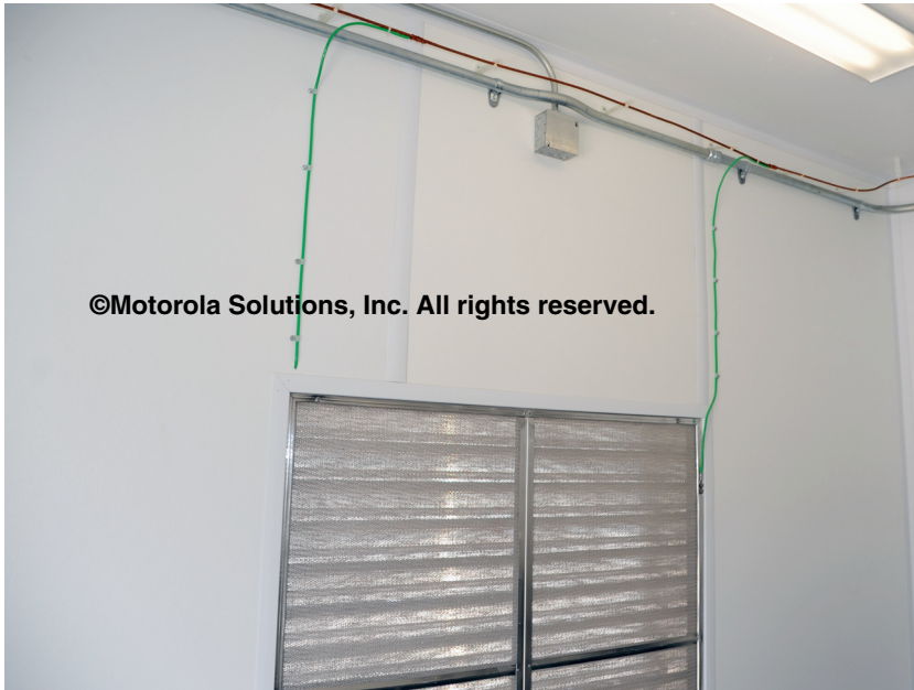
Figure 5-106 Example of Bonding Fresh Air Vent for Generator Room to Internal Perimeter Bonding Bus
