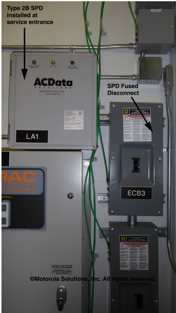
Figure 7-8 Example of Type 2B SPD Installed at Building Entry
