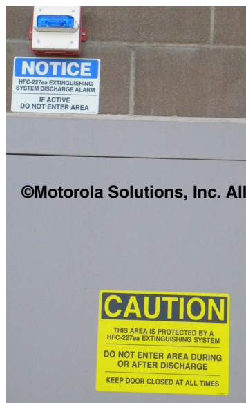
Figure 3-14 Example of Warning Signs
