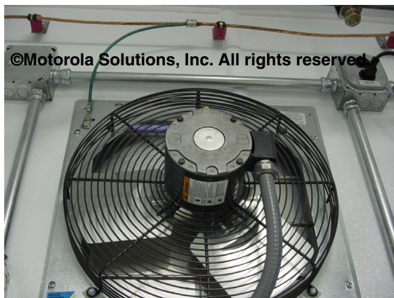
Figure 5-104 Example of Bonding Exhaust Fan to Internal Perimeter Bonding Bus
