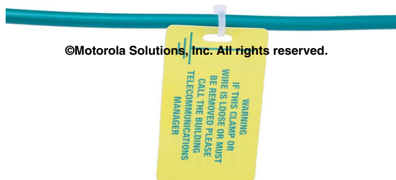
Figure 5-13 PBB Grounding Electrode Conductor Identification
