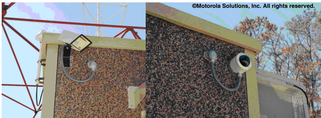
Figure 9-57 Securing and Protecting Surveillance Equipment Cabling
