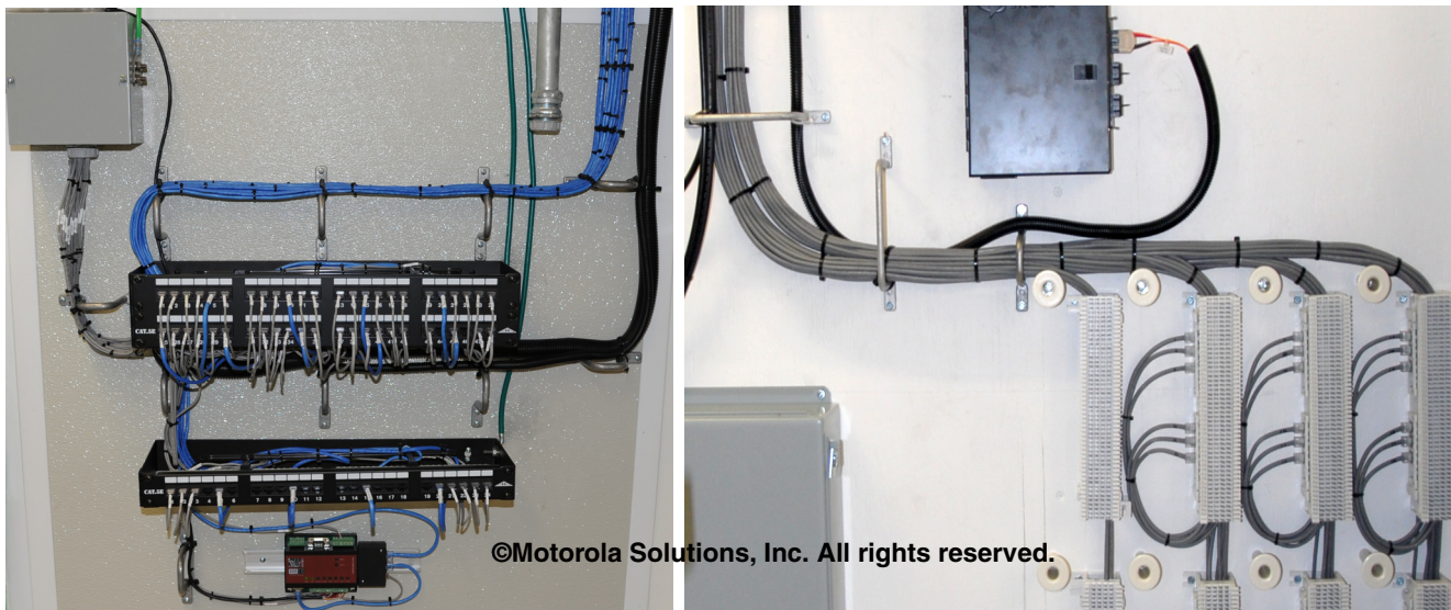
Figure 9-49 Examples of Typical Distribution Frame
