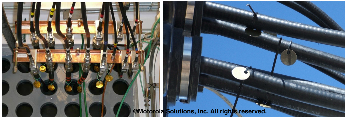
Figure 9-52 Examples of Interior and Exterior Cable Labeling
