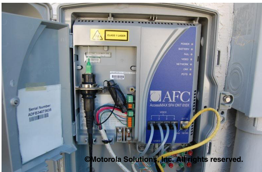
Figure 7-17 Typical Carrier Optical Network Terminal
